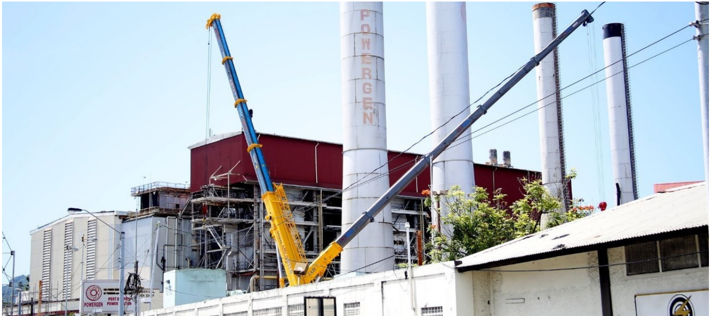
POWERGEN Port of Spain Power Station
